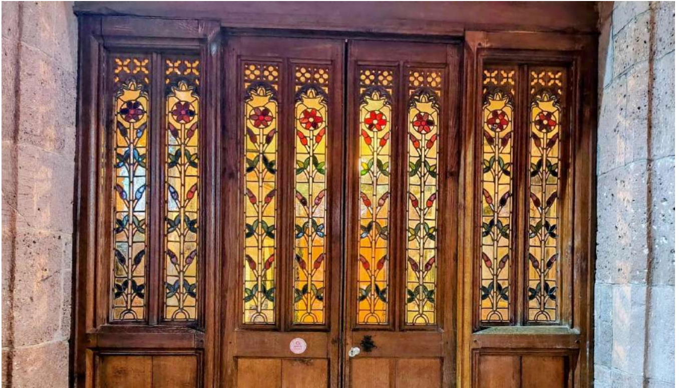
The glass in the tower vestry doors at Upton Pyne church was cracked and blown and looking dull. Fundraising from The Friends of Upton Pyne events and a grant from Devon Historic Churches Trust have enabled the glass to be fully restored to its former glory and sparkling from a good clean by Maggie!
